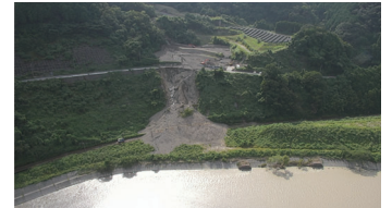
▲Tropical Storm Talas, September 2022 National Road 473 collapse(Fukuyo area)
